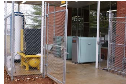
Curtis Wright – Sauer USA - WP4325 nitrogen gas compressor(s)
