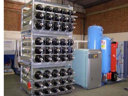
MSS – Sauer UK - WP4325 nitrogen gas compressor 350 bar
